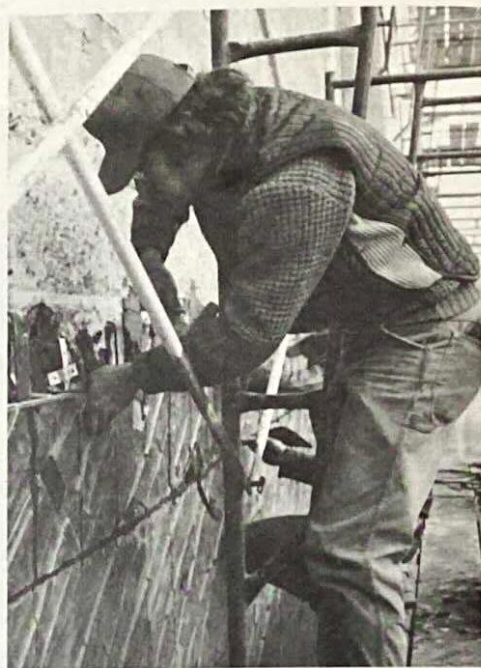
Both Greg Hardy and Randy Woolsey took an active part in the installation of their mural on the east wall of the Sturdy-Stone Centre. Here, Hardy makes sure the tiles are secure before moving on to another section of the mural. (Photo courtesy of the Government of Saskatchewan).
